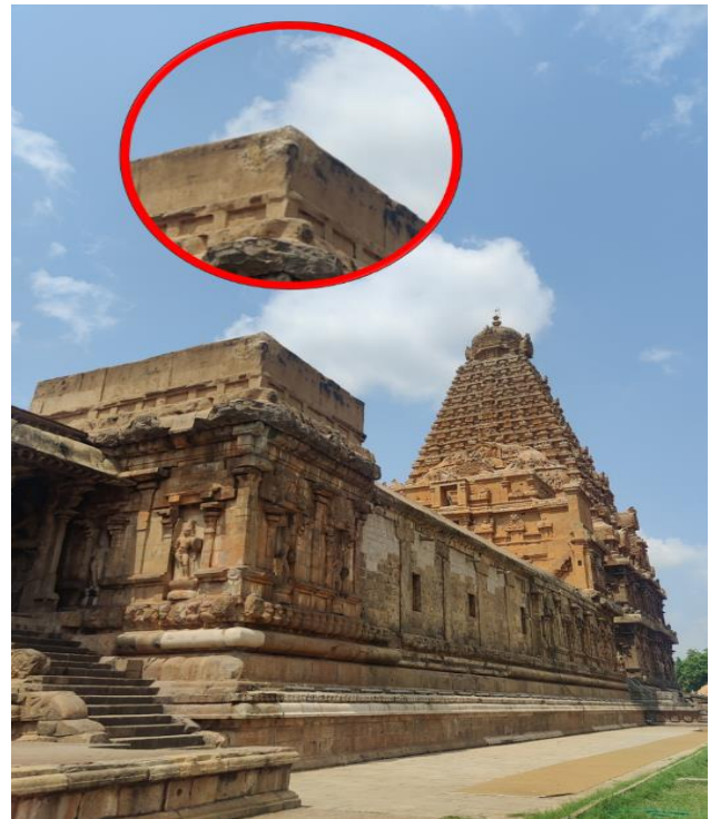
Figure 7: A Photograph of Brihadeeshwara temple located at the bank of the Cauvery river in Tamilnadu India. Shown in the inset is the edge of the temple that was struck by lightning.
