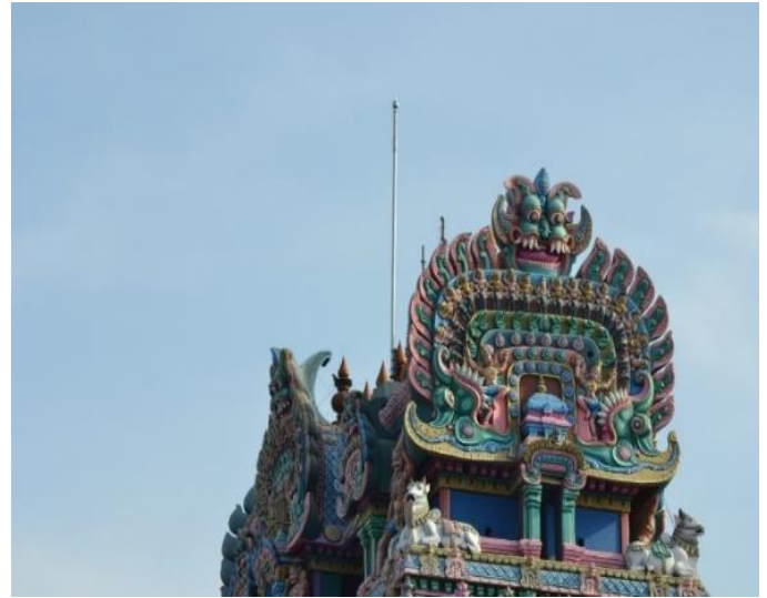
Figure 10: The ESE air termination system installed on the top of the building of Thiruvanaikaval temple.
